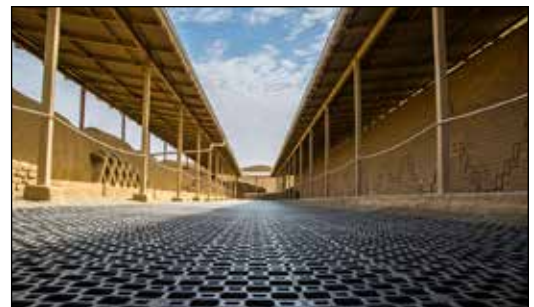
Installation of Atlantis Gravel Cell® at the Chan Chan UNESCO world heritage site.
