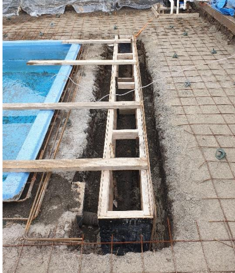
N12 rio in all walls & corners top and bottom Timber brace attached to formwork and pool edge to stop movement during concrete pour
