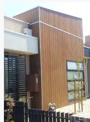
4 MONTHS: The board shows signs of lightening.
