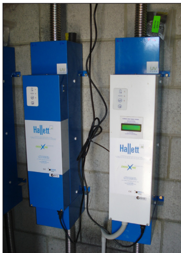
Hallett disinfection units for tertiary treatment.
