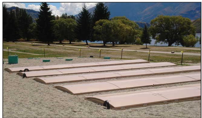
The facility features five Orenco® AX-Max units that employ the AdvanTex® recirculating media filter technology. AdvanTex units produce high-quality effluent with substantial reduction of nutrients, making them well-suited for any project with strict discharge limits.
